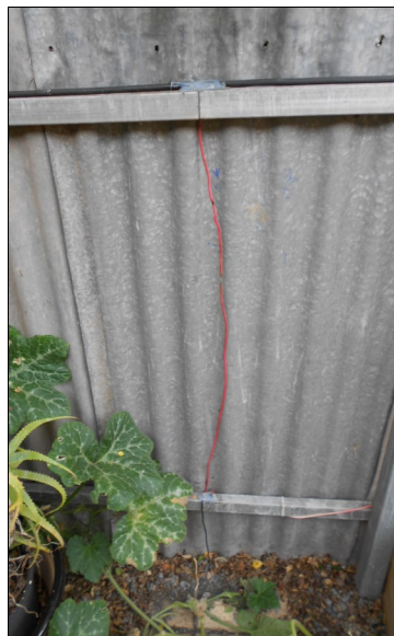
← Shows fence iron sheets and both metal fence rails bonded together with copper wire bridges.
