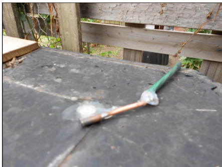
← A rain water tank bonded to a short radial at the aerial base.
